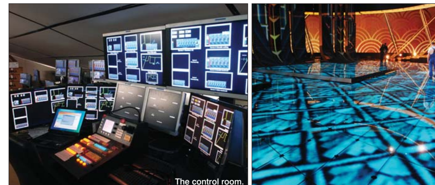
The control room.
